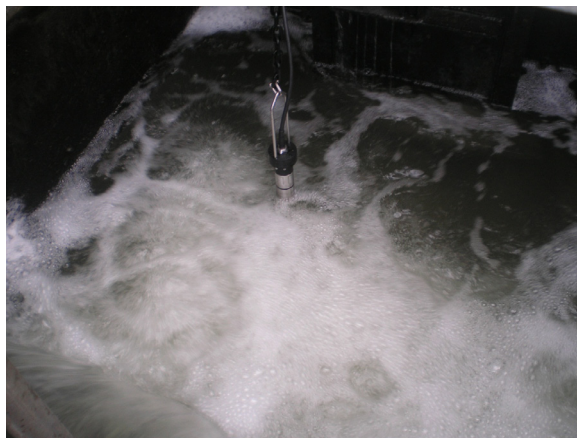
Figure 2: IQ SensorNet VARiON Sensor in Final Effluent
