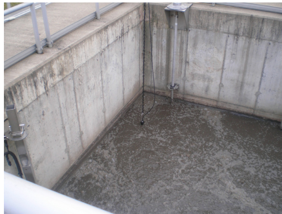
Figure 1: IQ SensorNet VARiON Sensor in Anoxic Tank
